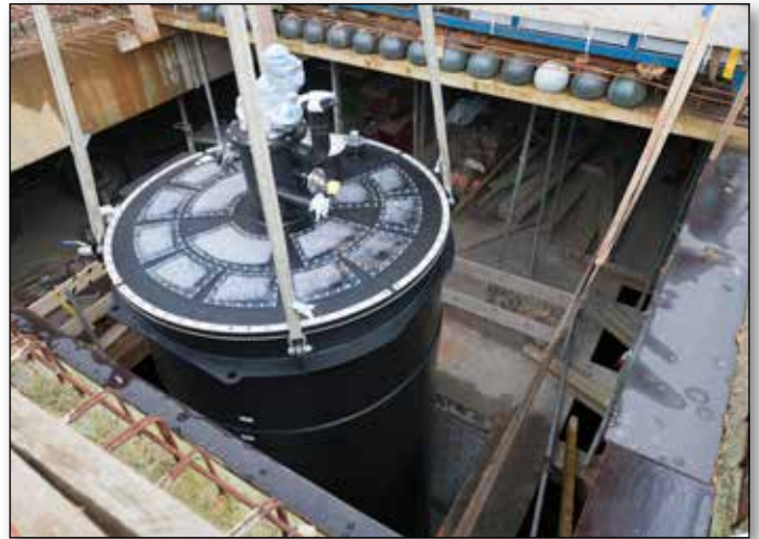
installation of black water reactor for a government office building in The Hague, NL
